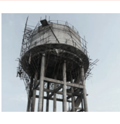
Water Storage Tank
