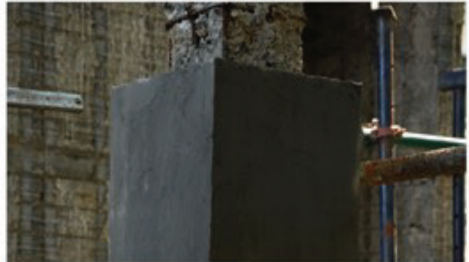
Remove the jacketing/Foam work after 24-48 hours and water curing or as per site in charge's instruction
